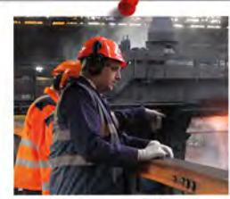
Steelmaking returns to Teesside with plans for a new electric arc furnace by British Steel currently underway.
